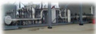
Mobile Injection, Dissolution & Dilution System
