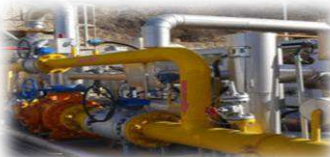
Gas Gathering Skid
