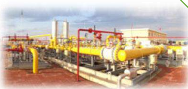
Skid-mounted Pressure Reduction Metering Station
