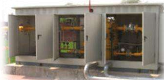
Skid-mounted CNG Pressure Reducing Station
